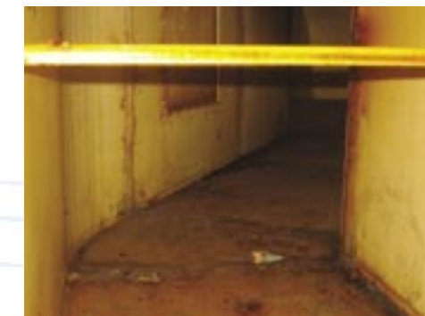
Horizontal main (grease) exhaust duct of the system with no UV equipment. Despite the regular stream wash the duct is clearly affected by grease. Grease accumulation existed in duct supports, brackets and fire detectors.
