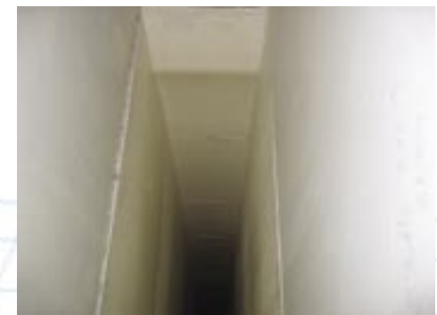
Vertical, white painted, main galley (grease) exhaust duct equipped with UV system. The duct is clean without any evidence of grease.
