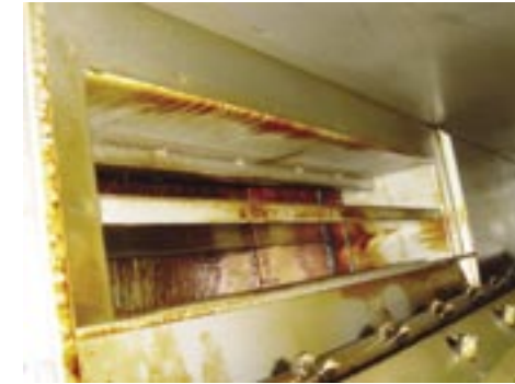
Hood fire damper a galley hood with no UV equipment. The damper is clearly covered with grease. The fusible link is completely covered in grease.
