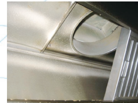
Interior of a hood fitted with KSA filters 18 months after installation.
